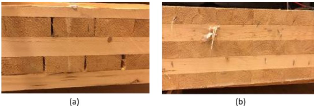
Figure 4.9: (a) Air gaps in the laminate layers of CLT. (b) No edge-bonding of CLT.
