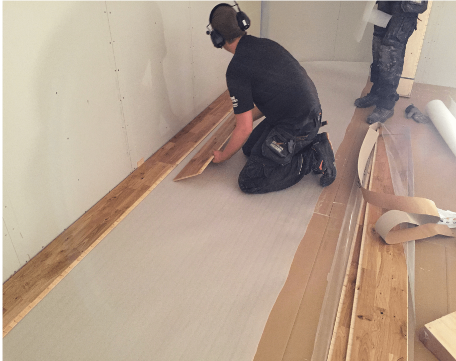
Figure 4.8: Topping floor installation using a parquet layer and underlying sheet in Luleå.
